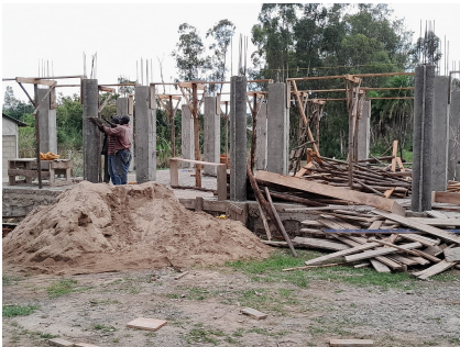
Construction in Kenya of the mission school housing. Above this will be women's dorms.
